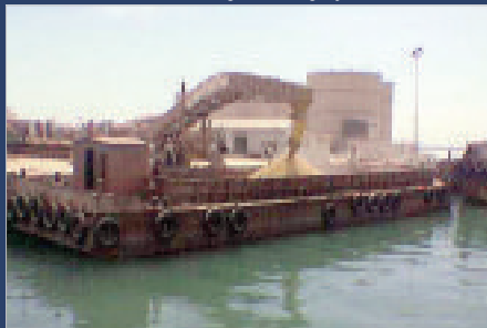
▲ 450 TPH Mobile Barge Loading System.
