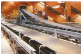
Belt Conveyor with travelling tripper.
