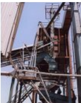
Ducting of dust collection system incorporated with coal handling system to make system totally dust free.
