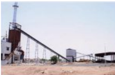
15 TPH coal/lignite processing & handling system with pre-screening arrangement at Gokul Overseas Gandhidham.
