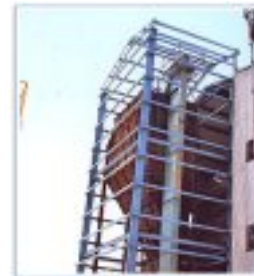
Bucket Elevator handling coal.
