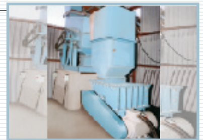
Primary vibratory screen feeding crusher in coal handling system with pre-screening arrangement.
