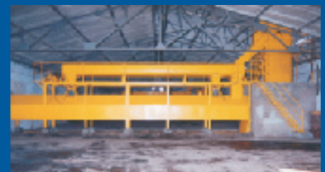
Godown feeding and reclaiming system (under ground) with 100 TPH capacity.
