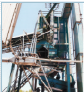
Ducting of dust collection system incorporated with coal handling system to make system totally dust free.
