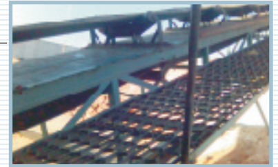
Close-up view of belt conveyor showing, belt, troughing idlers, deck plate, grating & bridge type structure.
