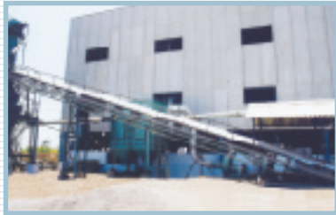
Inclined feed belt conveyor with bag filter in the background.
