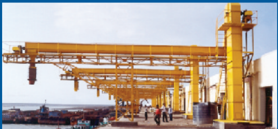
1000 TPH Barge loading infrastructure at Bedi Port, Jamnagar.
