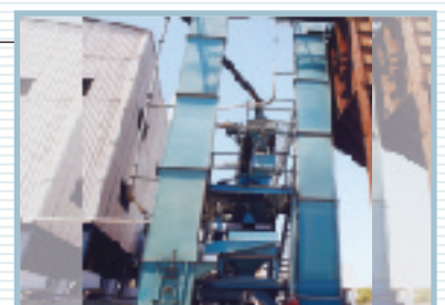
View showing recycling bucket elevator feeding crusher and product bucket elevator feeding bunker.
